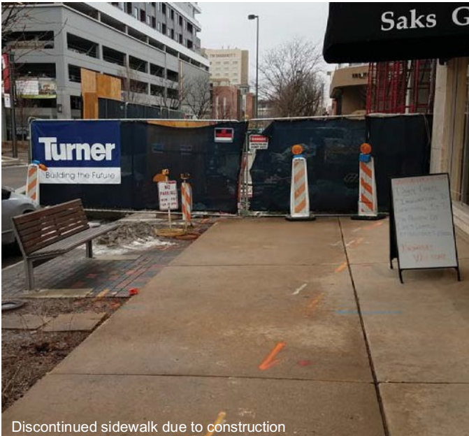
Discontinued sidewalk due to construction
